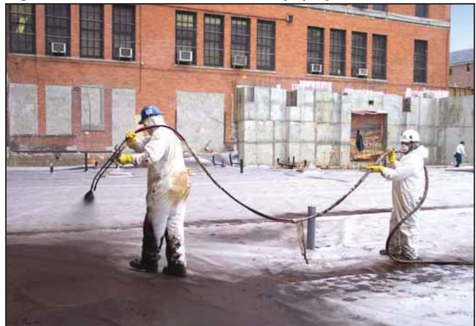
Figure 2. Installation of a fluid-applied vapor barrier at a public school in Queens, NY.
